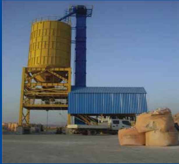
Fly Ash storage & Handling System
